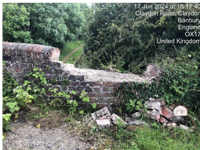
Figure 2-12: Section of damaged parapet [2024].
