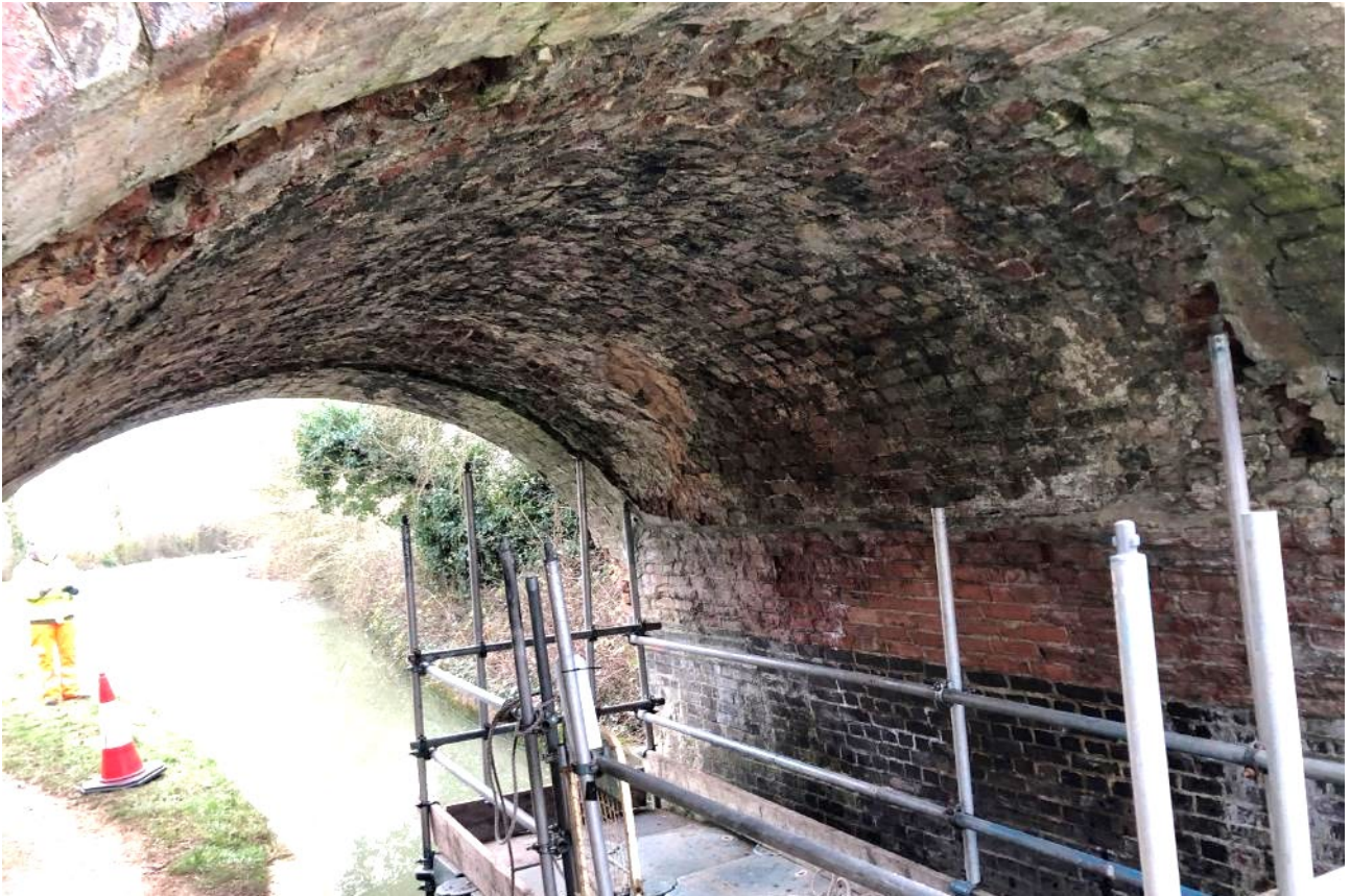
Figure 2-2: Intrados of arch barrel, historic repairs in stretcher bond visible above the blue brick abutments on the right of the photo [2024].
