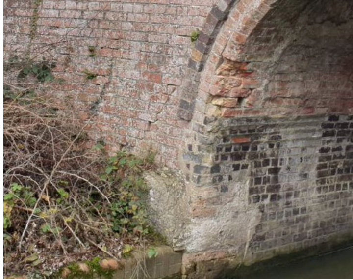
Figure 2-10: South-west springing and wingwall showing stepped cracking in brickwork [2022]
