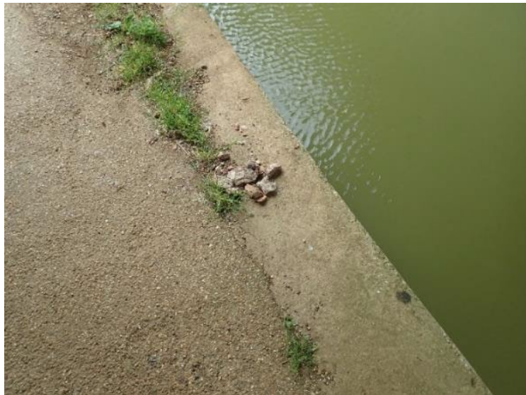
Figure 2-3: Evidence of dropped material from the intrados [2019].
