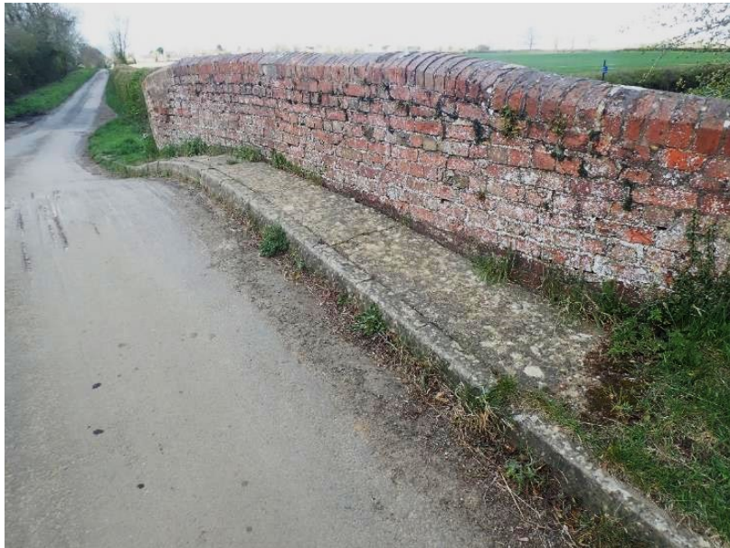
Figure 2-11: Parapet over the structure (prior to damage in 2024), concrete verge, and carriageway with undercarriage scraping marks [2021]
