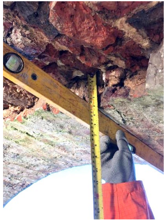
Figure 2-5: 95mm spalling depth measured at north end of arch barrel near crown [2024].
