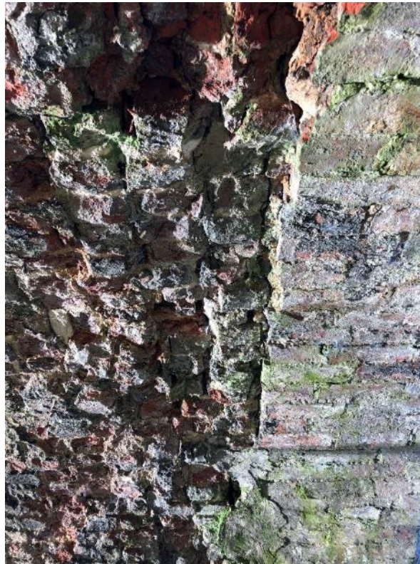
Figure 2-1: Photo of arch barrel close to north elevation along interface between voussoir and main arch barrel section [2024].
